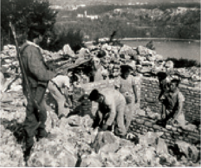
Sailors building a fortified look-out in the same area as the previous photo.
